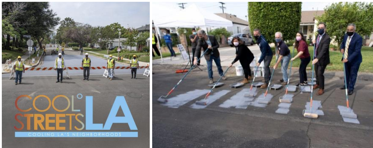
Figure 2: StreetsLA reflective coating trial applications using GAF Streetbond Durashield Cool pavement coating
