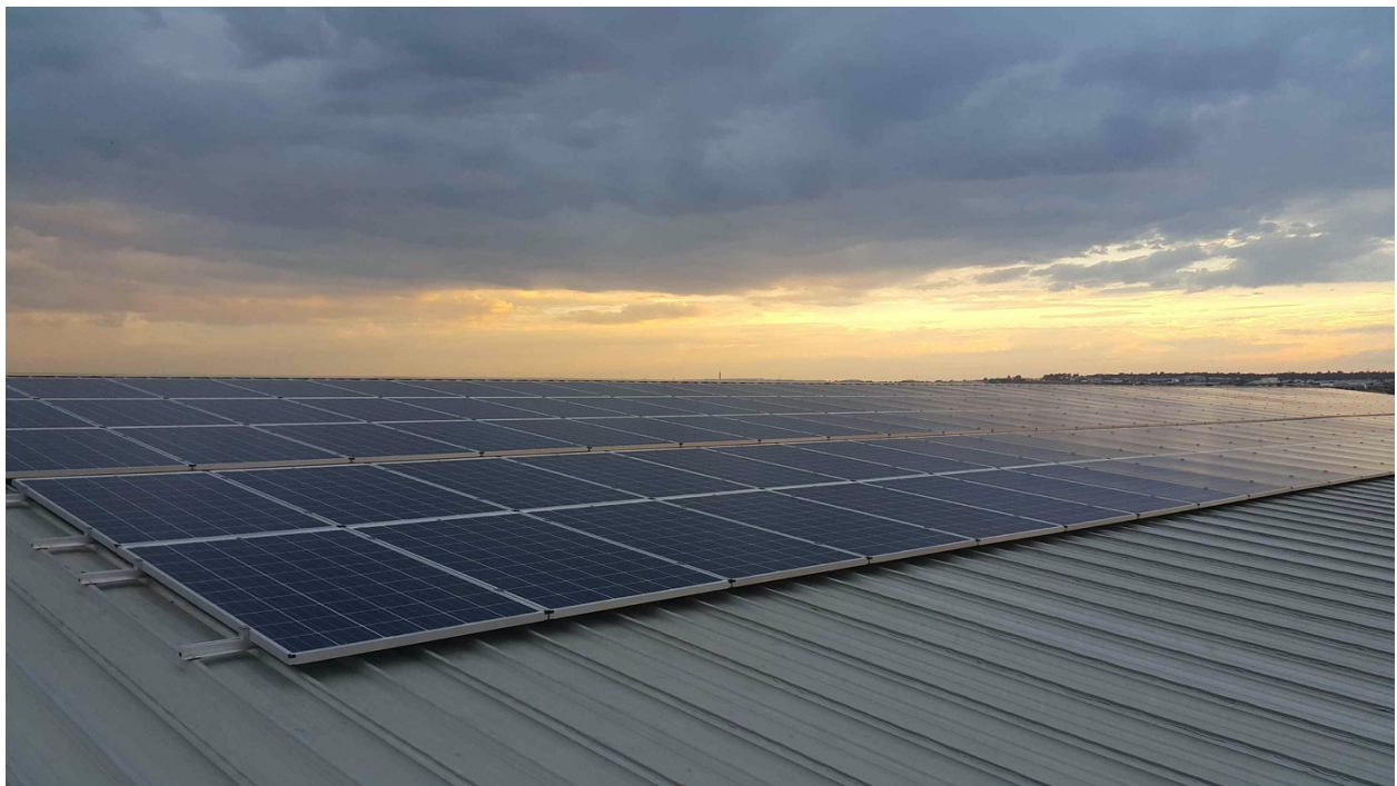
Figure 7.7. Example of Solar PV.
